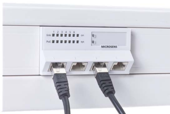
GBE G6 switch installed in MS140090
