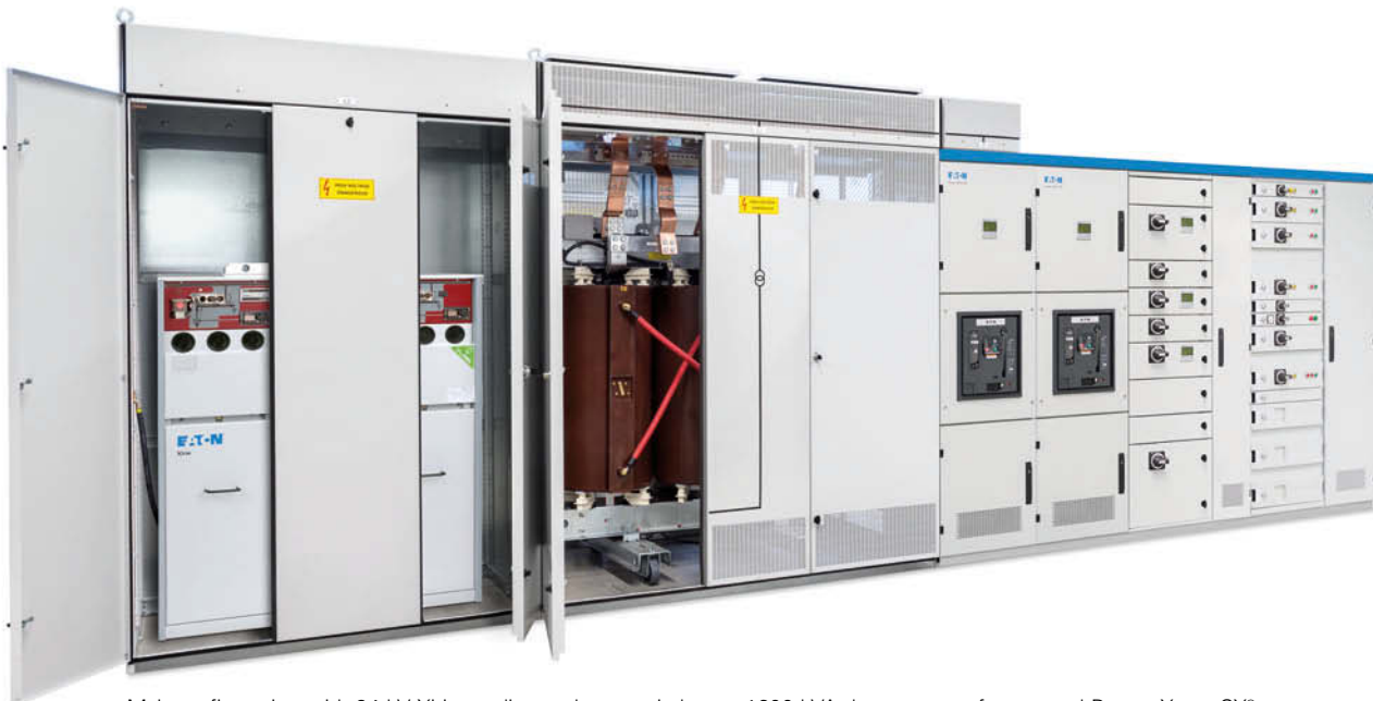
M2L-configuration with 24 kV Xiria medium voltage switchgear, 1600 kVA dry-type transformer and Power Xpert CX®.
