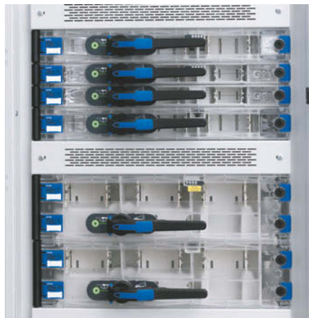
Form 3b compartment with fused switch-disconnectors.
